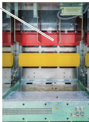
Shutters closed (VCB)
