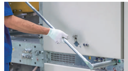
Earthing switch operation
