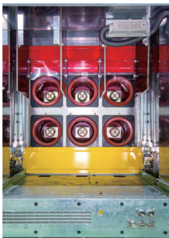
Shutters open (VCB)
