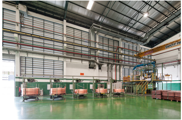
Up-Casting Introduction Furnace
